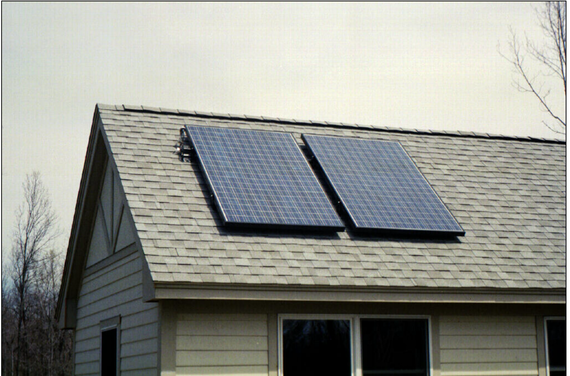
Photovoltaic modules: Pathways Co-housing in Northampton, MA
