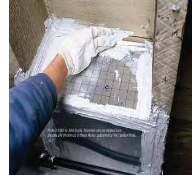
Tight Construction and Ducts
