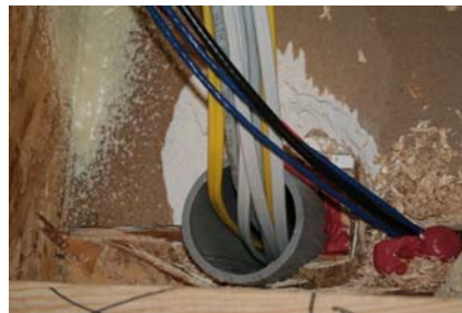
Wiring chase ways should be sealed.
