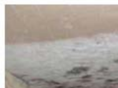
MOLD: When warm air leaks, condensation can occur. This mold compromises the structure.
