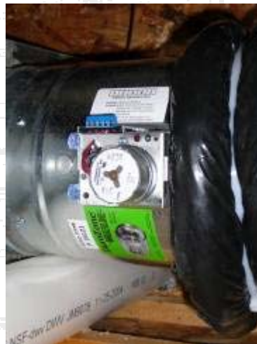
FRESH AIR DAMPER
