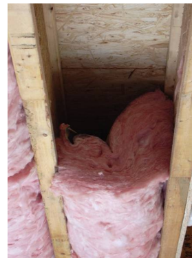
Insulation settling away from sub-floor
